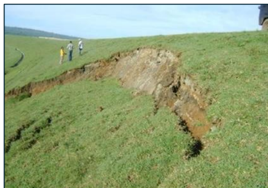
Figure 1 Slide of the downstream slope, Cuban-Bulgarian Friendship Dam.
